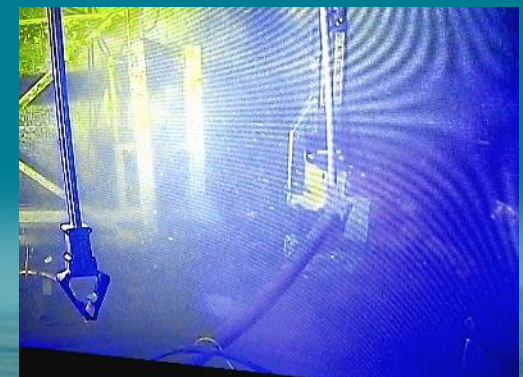
Long-reach cutting tools are used to cut hoses in the K West Basin for sorting and staging on the basin floor. – December 2022
