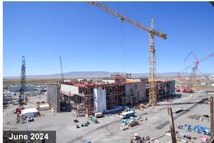
June 2024 High Level Waste Facility
