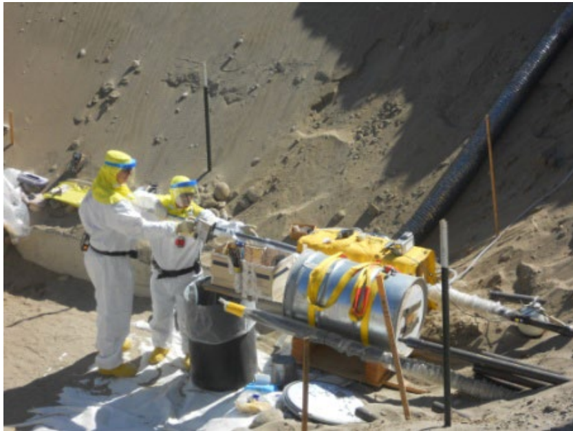
Piping is driven beneath the building foundation to collect soil samples and radiological readings
