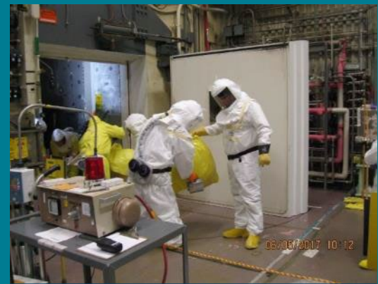
Workers dressed in protective clothing remove waste from a hot-cell airlock for disposal.
