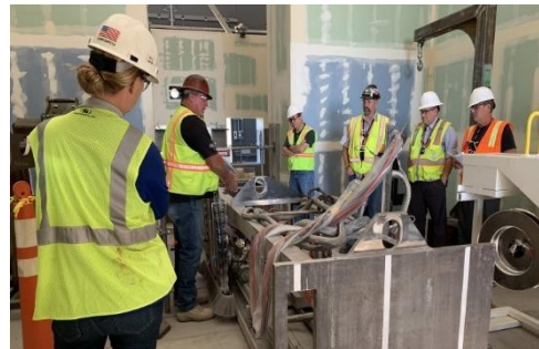
Workers installed and tested a saw at the mock-up, which will soon be installed in B-Cell to cut through the concrete floor.
