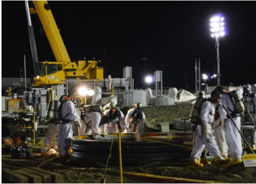
A/AX Tank Farms at night
