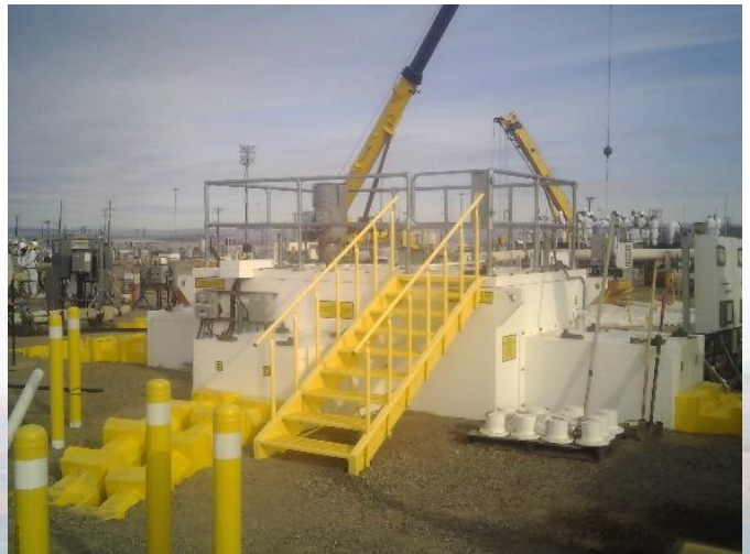
Portable valve boxes installed in AX Tank Farm
