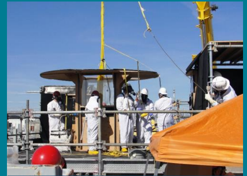
Shield box for Tank AX-103.
