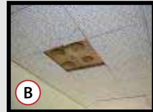
Asbestos Ceiling Tiles
