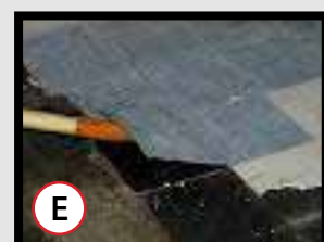
Asbestos Floor Tiles
