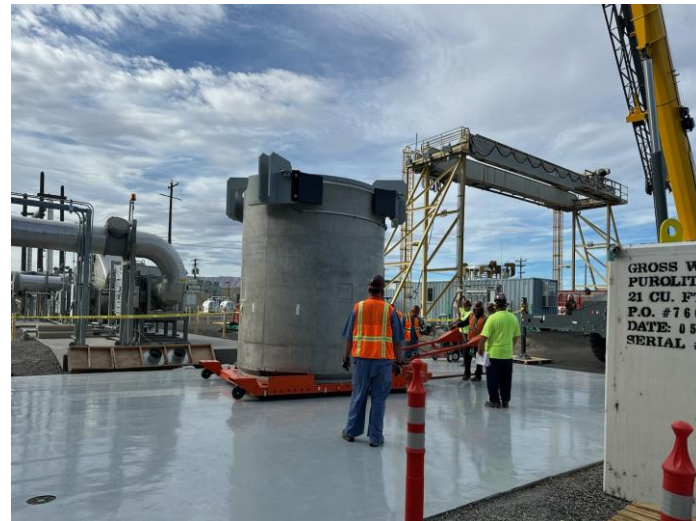
Waste Encapsulation and Storage Facility equipment testing
