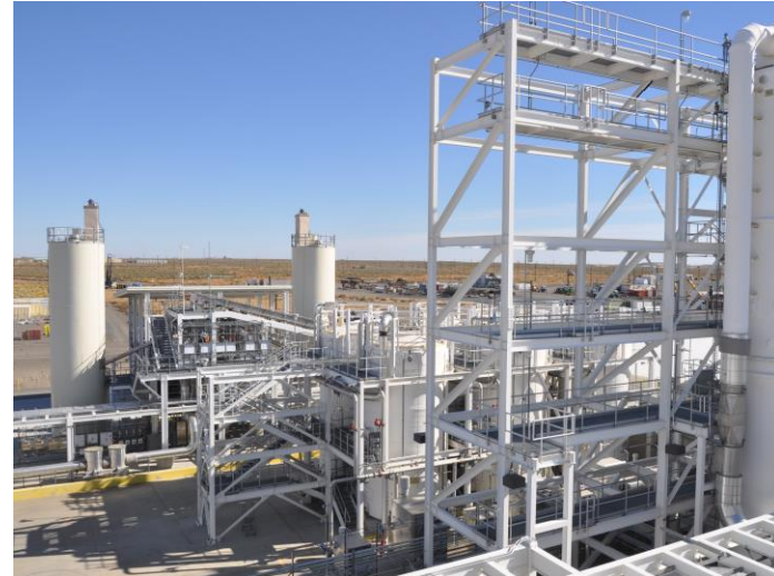
Groundwater treatment expansion
