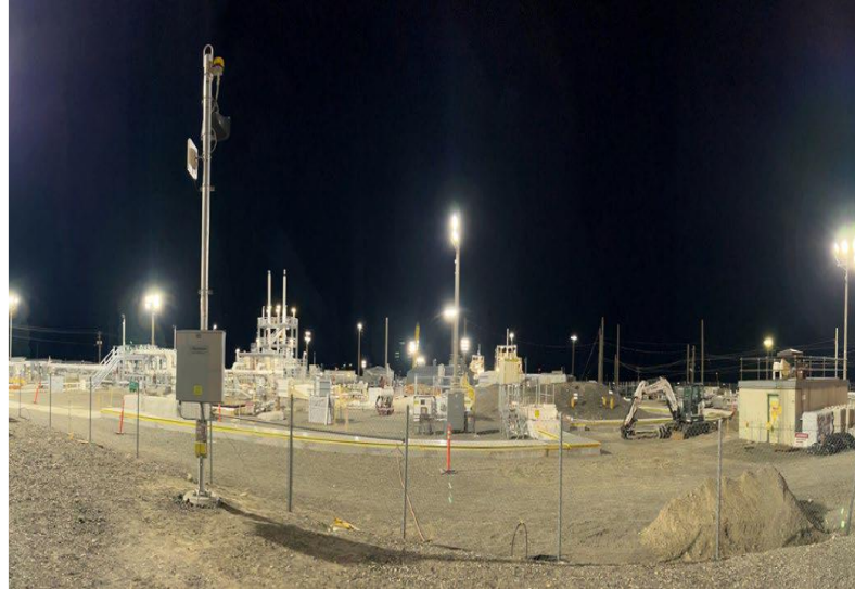
A Tank Farm is the third set of tanks to undergo waste retrieval
