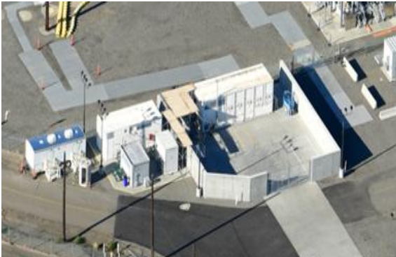
Tank-Side Cesium Removal System
