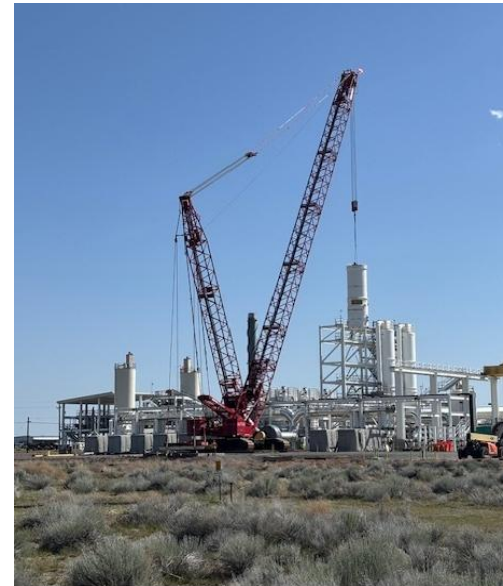
Groundwater treatment expansion
