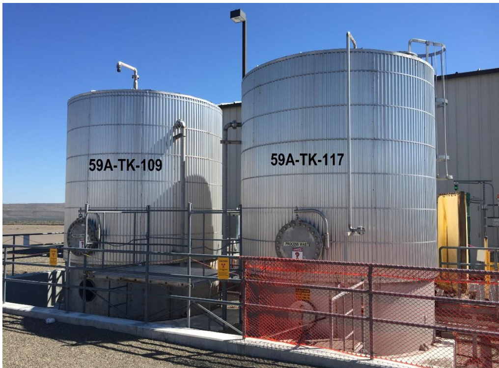
Load-In Station Tanks (59A-TK109 and 59A-TK-117) located next to Building 2025-ED.
