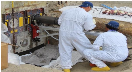
Upgrades are underway to the transfer lines that connect the 242-A Evaporator to the 200 East Area tank farms
