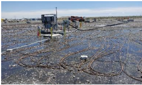
Soil flushing was initiated near the former K East Reactor in June 2022 to expedite the cleanup of hexavalent chromium.
