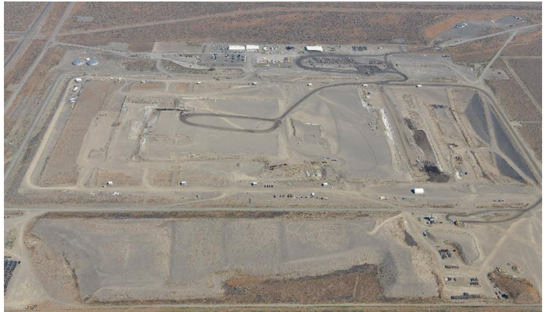
Workers are scheduled to construct a new disposal cell at the Environmental Restoration Disposal Facility to support ongoing cleanup activities across the Hanford Site.
