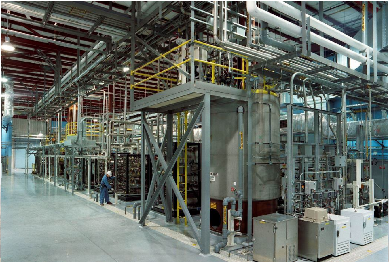
A worker inspects the main treatment train on the process floor of the Effluent Treatment Facility.
