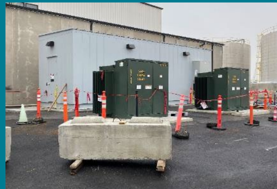
An additional electrical house was added to provide power to new facility infrastructure needed to support direct-feed low-activity waste operations.
