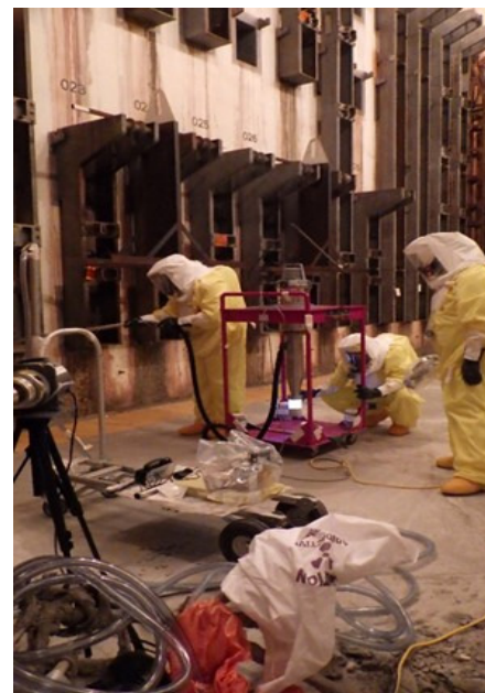
In March, after pouring a protective layer of grout on the floor to limit employee exposure to radiation, workers began vacuuming contamination from the Plutonium Reclamation Facility canyon.
