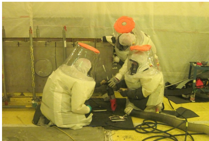
Workers at the PFP used enhanced personal protective equipment, known as "Level B" suits, during cleanup of highly hazardous areas in the plant
