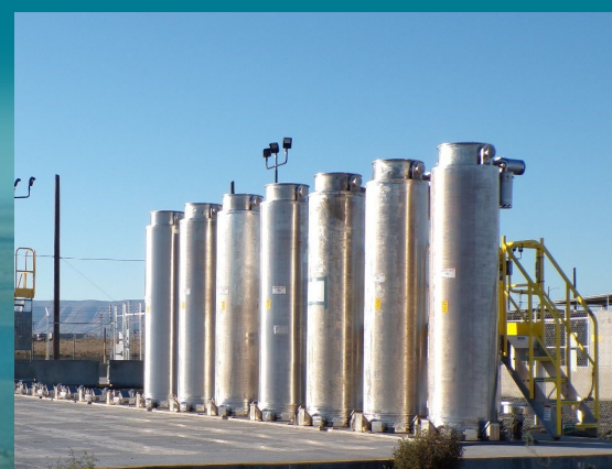
Spent ion exchange columns on the Tank-Side Cesium Removal System storage pad.
