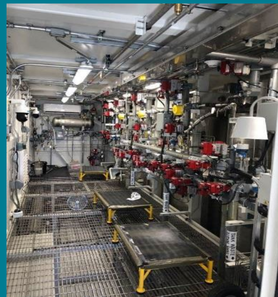
Inside the Tank-Side Cesium Removal System.
