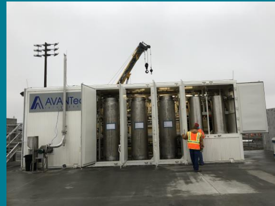
Tank-Side Cesium Removal System enclosure with the bay doors open.
