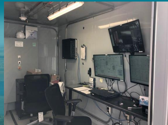
The system control room.
