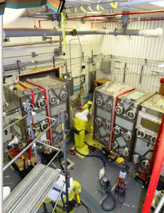
Separating Glovebox HC-230C-3 in Room 230C
