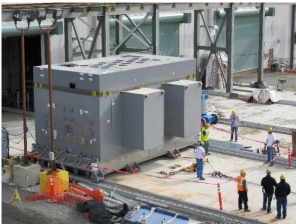
In 2012, a Low-Activity Waste Facility melter is pulled out of the building on rails for inspection. The melter will be one of two used to heat Hanford's underground low-activity tank waste and glass-
