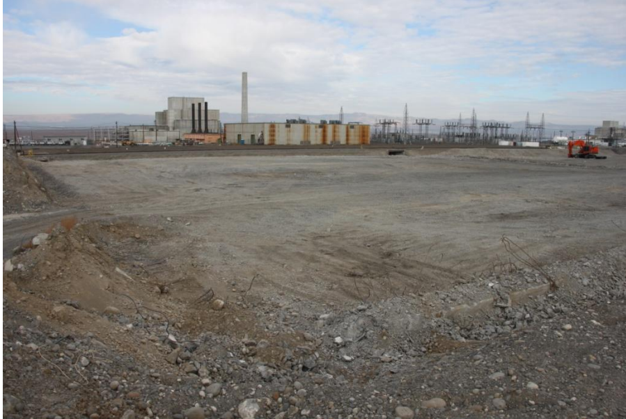
The 183K West Sedimentation Basin during demolition. CH2M HILL workers have completed demolition of the large 290,000 square foot structure.
