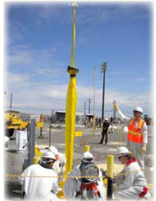
Employees of Federal Engineers & Constructors (FE&C), a locally based small business, modify instruments on a tank in AP Farm that will significantly increase the operating level of the tanks.
