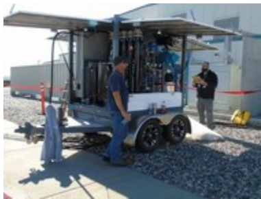
Mission Support Alliance substation electrician Matthew Starkey, left, and environmental compliance officer Mike Demiter perform oil reconditioning on a transformer.
